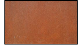
Heavy Textured Rust
