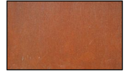
Heavy Textured Rust
