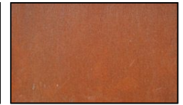
Heavy Textured Rust
